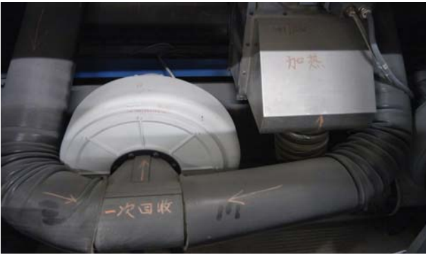
Printing Press equipped with Energy Recycling Functions
