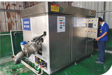
Low-temperature distillation and drying equipment
