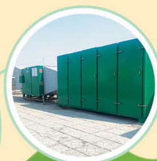
VOCs treatment system
